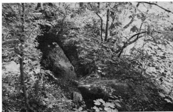
Mustapha Island Bridge, along Ohio Route 124, in Athens County. This span is formed in sandstone of Permian age.
